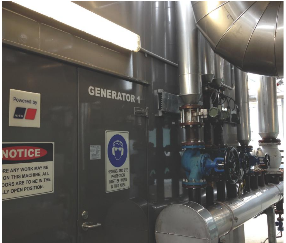
Right: The exterior of the soundproof enclosure that houses MTU Onsite Energy's GR 1169 N5 genset, featuring the 12V 4000 L33 engine, and the GR 1718 N5 genset, featuring the 16V 4000 L33 engine.
